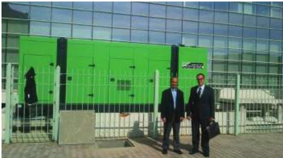
SEEI manager Mourad Najjar and Inmesol sales manager for Africa José María Hernández in front of the equipment installed in Carthagène International Hospital Centre
