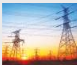
The new power line will establish Zimbabwe as a regional power hub. (Photo: zhengzaishuru/Shutterstock)
