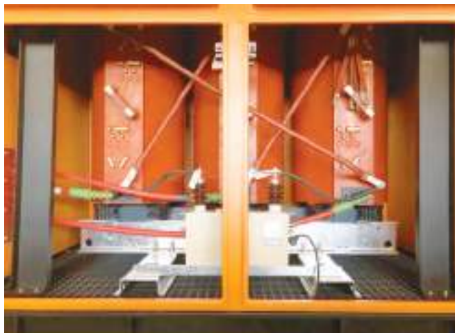
Cast resin transformer in fully enclosed mini-sub configuration.
