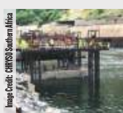
The first concrete pier set to float, which has a total length five metres.
