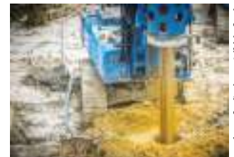
According to the company, the service allows rapid responses and minimises potential downtime on the project.
